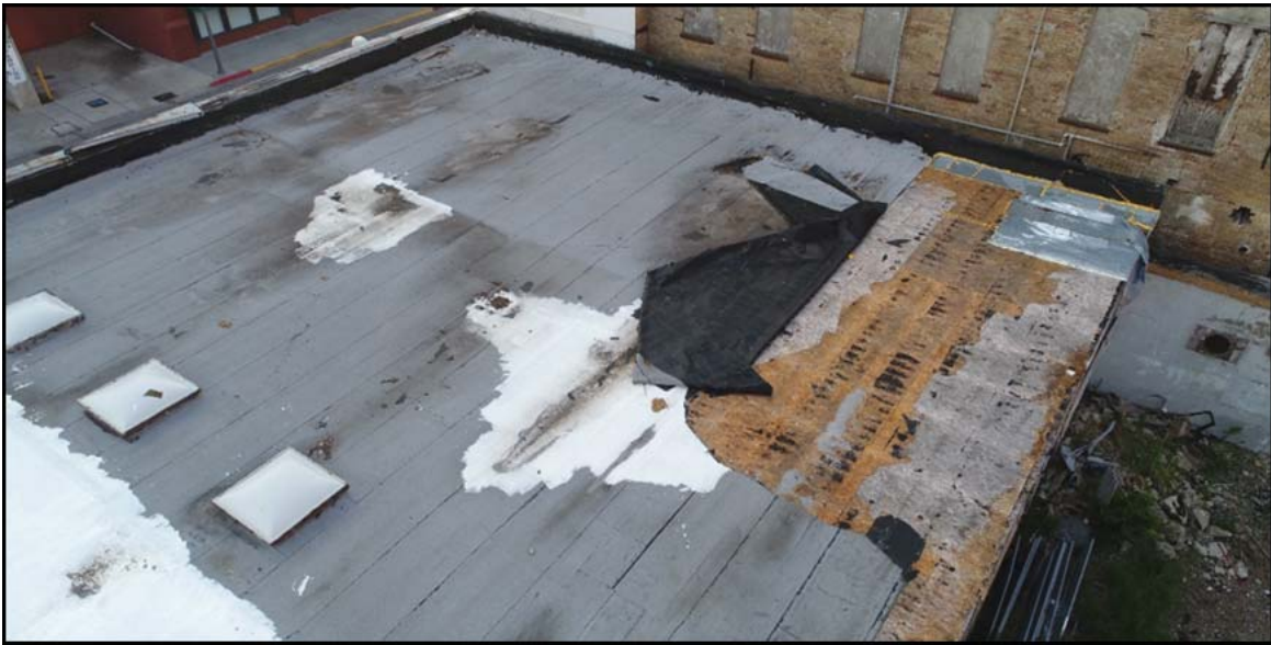
Roof deemed unsafe to inspect. A drone was the best and most timely way to inspect the damage.
