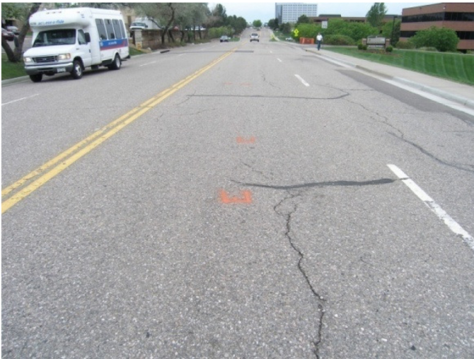
Figure 2. spray paint evidence- tire marks
