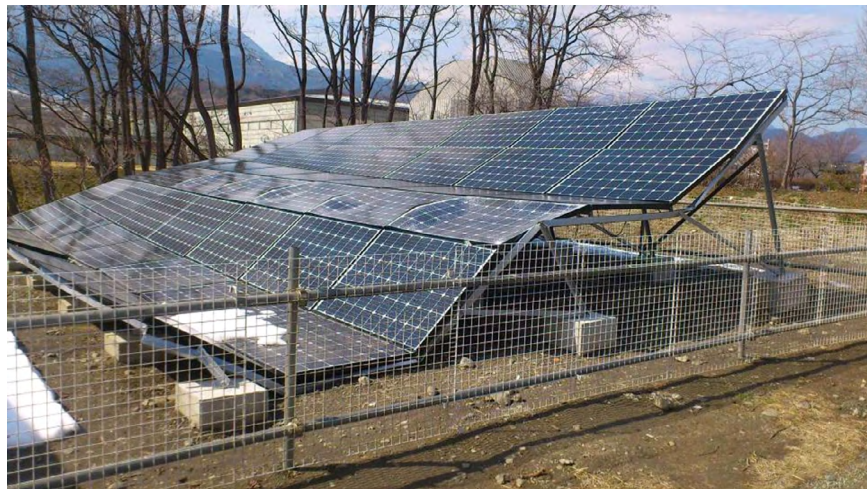
Figure 2 - Panels damaged from accumulated snow that has since melted away (Source: https://www.aquasoli.com/blog/snow-load-damages-reported-in-japan/ )
