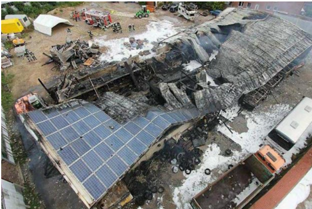
Figure 1 - Fire in a factory in Norderney Germany, 8/2013. Damage cost totaling millions of euros (IEA) (Source: https://solarity.cz/blog/fire-hazards-and-mitigation-in-photovoltaic-systems/ )
