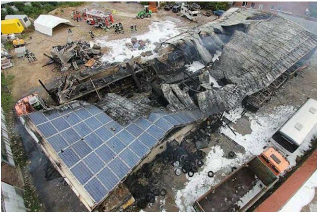
Figure 1 - Fire in a factory in Norderney Germany, 8/2013. Damage cost totaling millions of euros (IEA) (Source: https://solarity.cz/blog/fire-hazards-and-mitigation-in-photovoltaic-systems/ )
