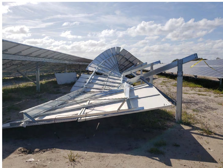
Figure 3 - The panels lying on their side in the background came off during a storm, were blown around, and were found in the water on the site. (Source: https://dailyhaymaker.com/coastal-nc-storm-damage-raises-even-more-questions-re-solar-farms/ )
