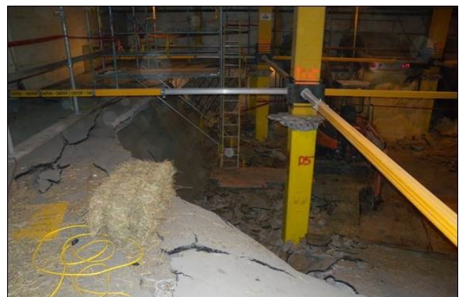
Figure 1 - Collapse of the upper level of the underground parking garage.
