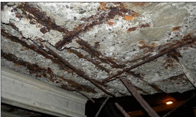
Figure 3 - A close-up of the underside of the concrete slab shows the severe corrosion of reinforcement rebars.
