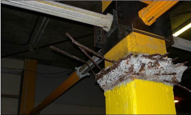
Figure 2 - Close-up of the column-slab connection shows the corrosion of reinforcement rebars.
