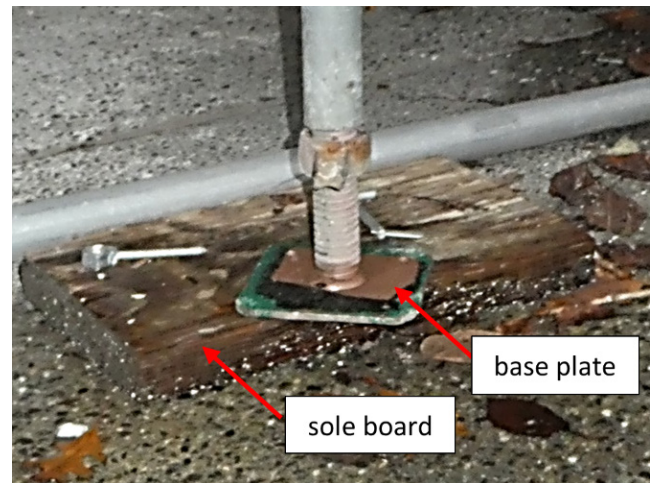
Figure 4 - Improperly positioned sole board.
