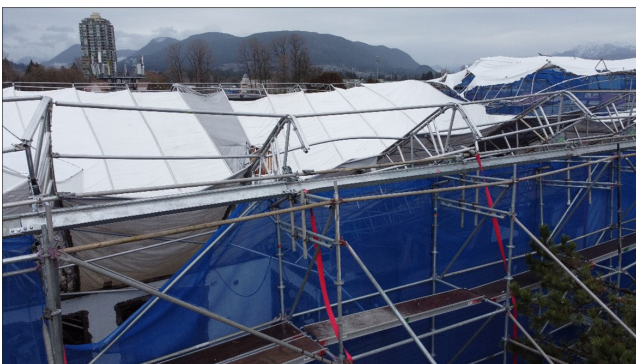
Figure 1 - A collapsed temporary roof structure supported by scaffold.
