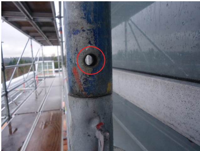
Figure 3 - Omission of scaffold locking pin.
