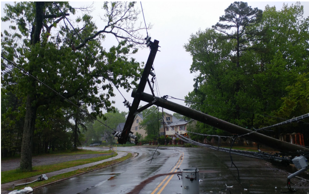
Figure 6 - Downed power lines resulting from a severe storm and high winds—common damage following tornadoes and hurricanes in the Southeast.
